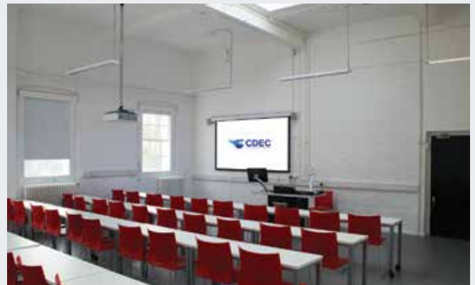
Six standard area types were defined when CDEC handled the supply and installation of AV systems across the Goldsmiths campus
