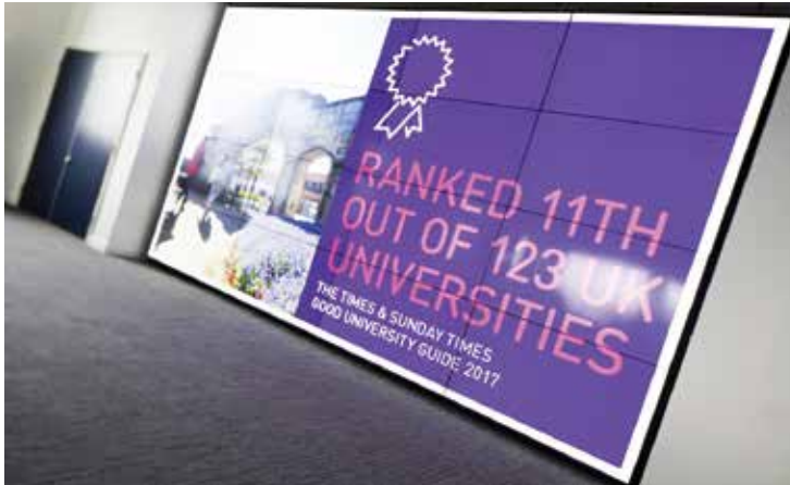
Integrator Pure AV installed this videowall for Loughborough University
